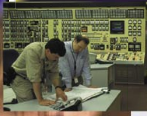
Operators man Georgia Power's Plant Vogtle nuclear power plant control room around the clock. The 2,320 megawatts capacity nuclear power plant is located near Waynesboro, Ga.
